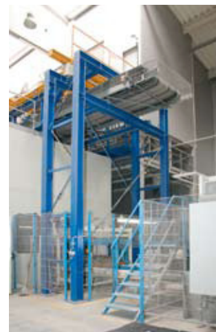
Fig. 6 Discharge on wet side and Colormix unit (above).
